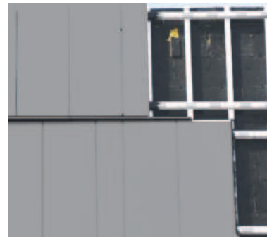
OPAQUE CLADDING (EW1C) Material: Precast and cast in place concrete Colour: Light grey Location: Exterior cladding on Ancillary buildings, EEB's
