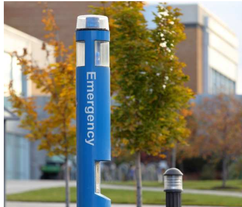
Figure 3-64: Exterior Emergency Blue Light Station
