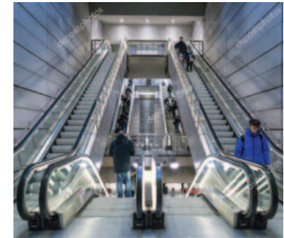
ESCALATORS/HANDRAILS WITH INTEGRATED LIGHTING
