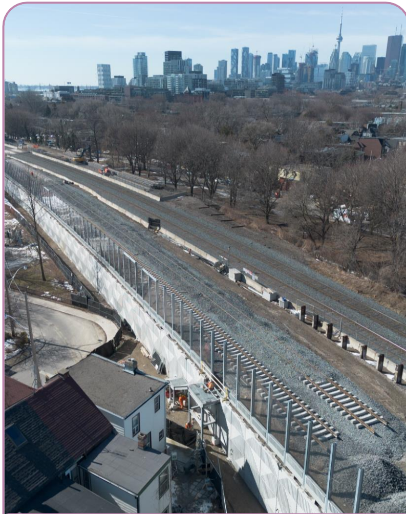
Completed retaining walls and noise barriers at Booth Ave. and Paisley Ave.
