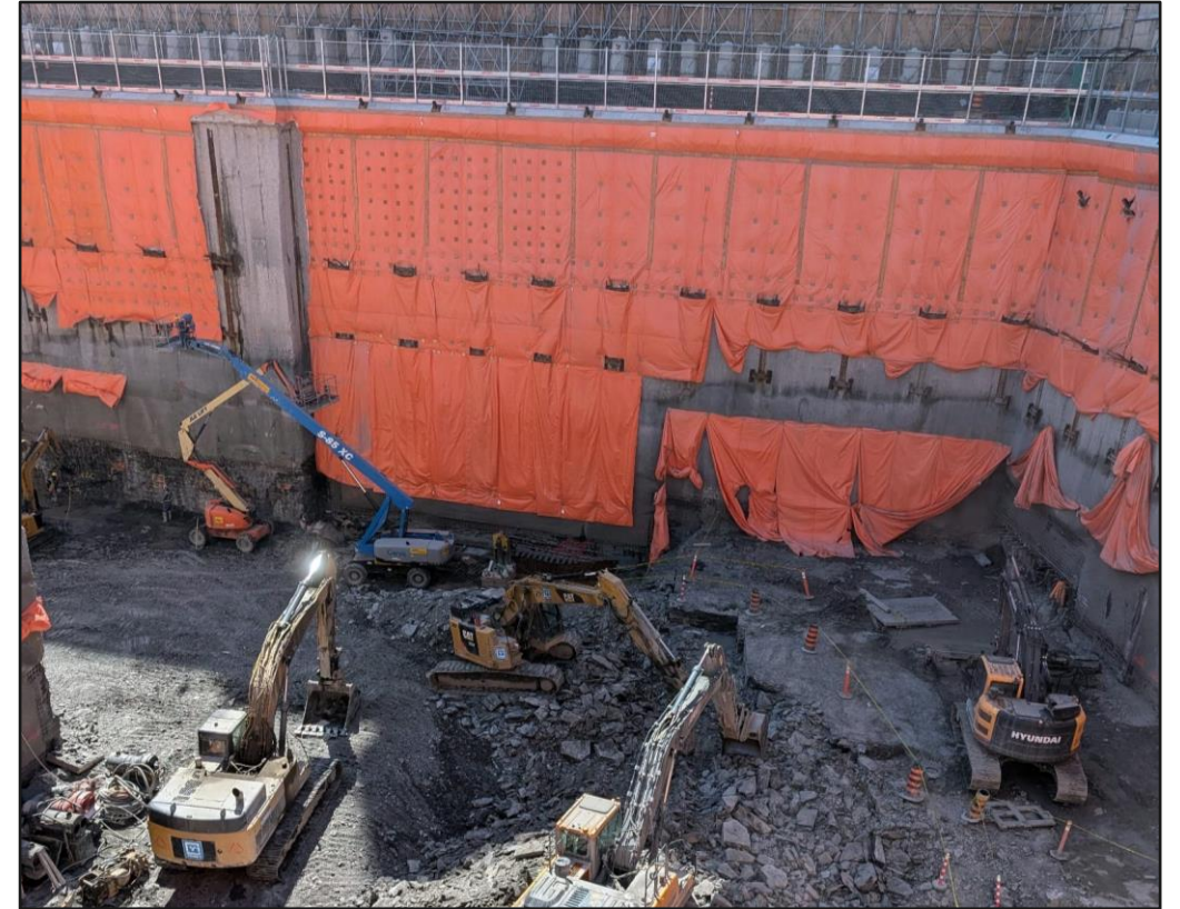
North shaft excavation at the northwest corner (King St. E. & Berkeley St.)
