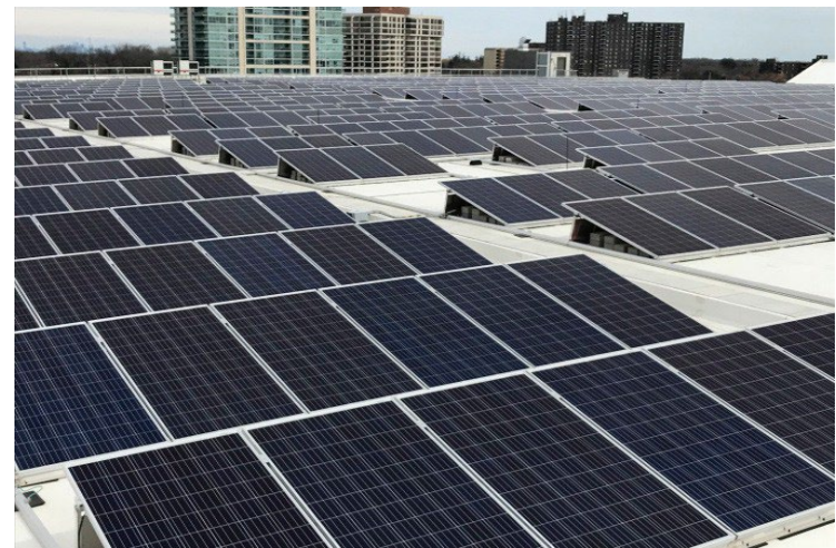
Figure 3: Erindale GO Station, 250kW, Installed 2013
