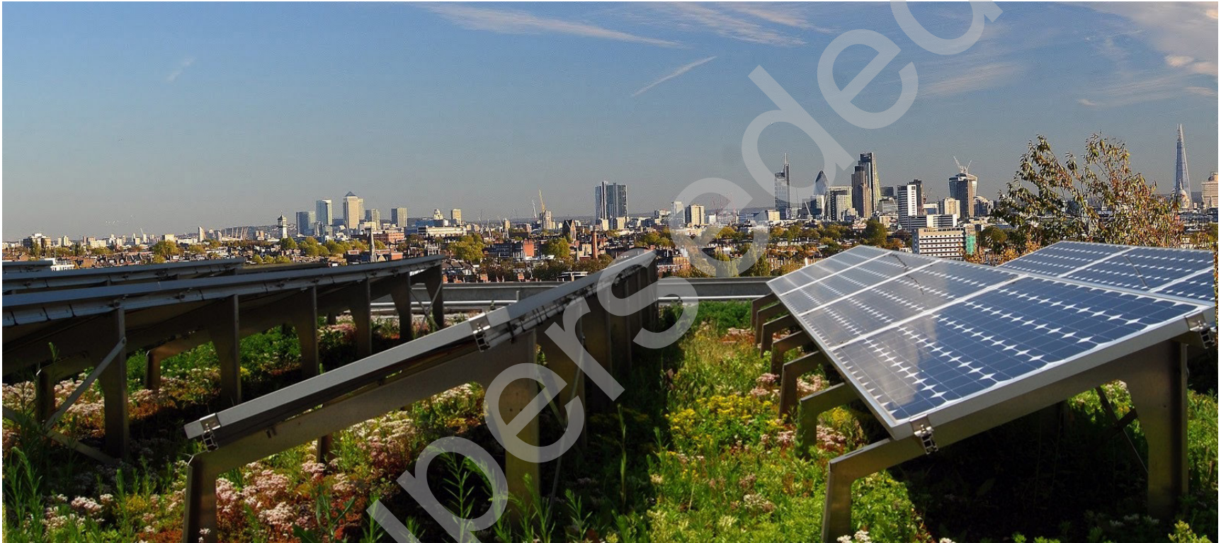
Solar Panels on Green Roof (Image Source: Greenwood at medium.com)
