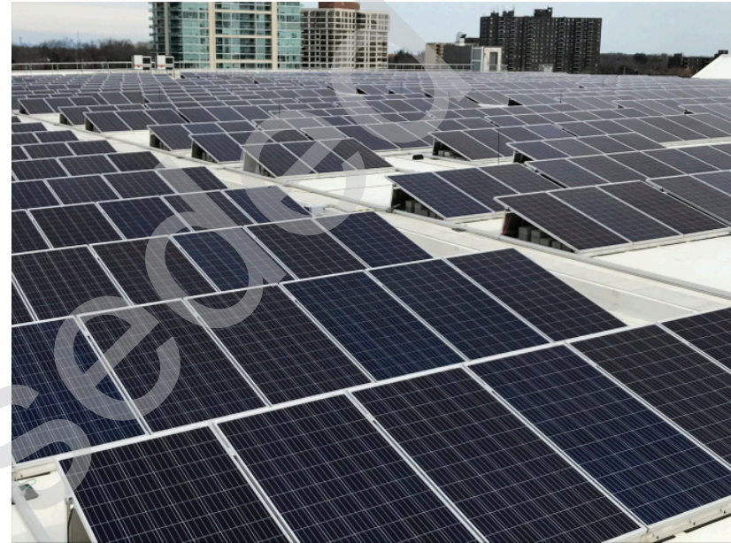
Clarkson GO Station. On top of the 1,500-space, five-storey parking structure, the roof is entirely covered with solar panels.
