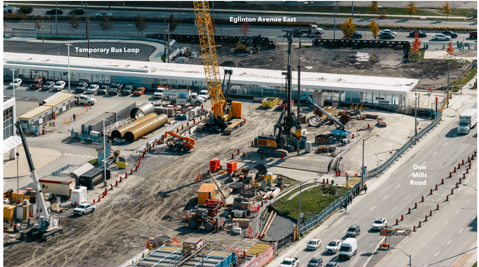
Looking south - Nov. 2, 2025
