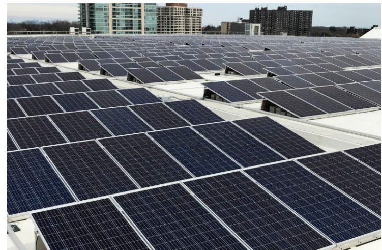
Figure 3: Erindale GO Station, 250kW, Installed 2013
