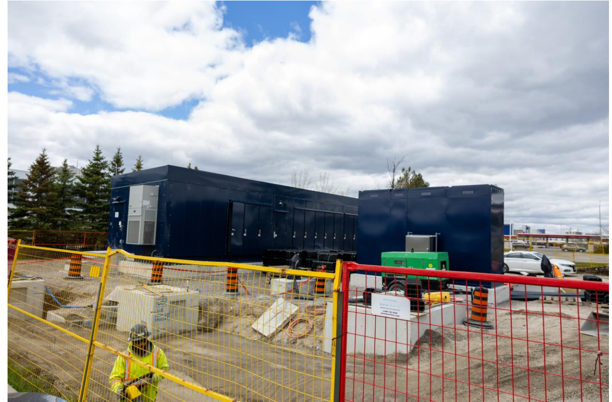
Traction Power Substation (TPSS) 14 located at Hurontario Street and Steeles Avenue
